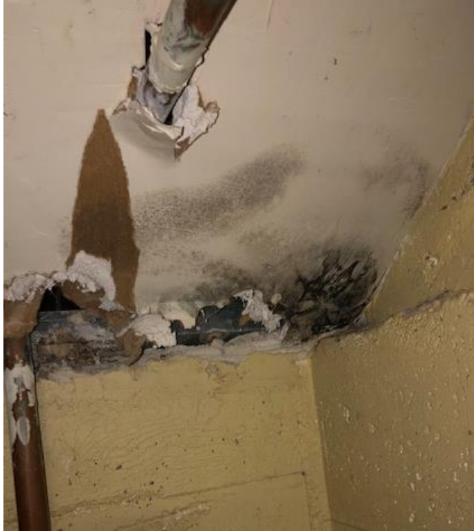
Figure 1: Mold on West stair well drywall.
